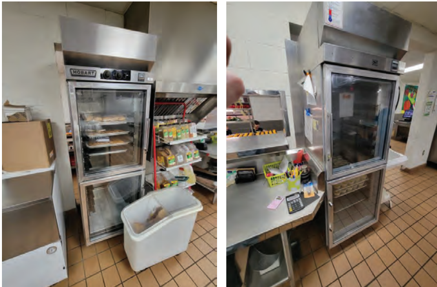
The pass thru refrigerators and heated cabinets have reached their life expectancy and are in need of replacement.
