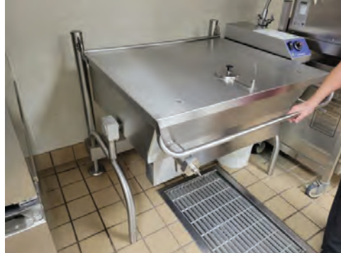
The handle for the tangent draw on the braising pan is missing.
