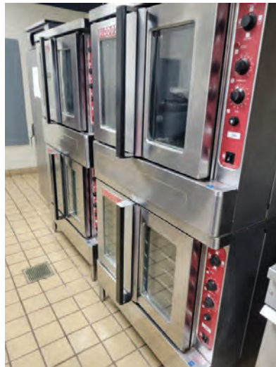
Staff recommended replacing one convection oven with a combi oven.
