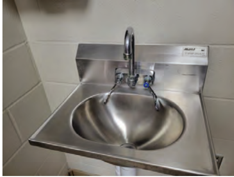
The faucet on the hand sink next to the cooking line is not functional.
