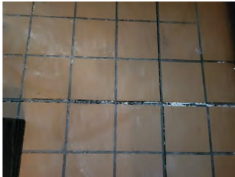
The quarry tile floor on the interior of walk-in cooler and freezer is showing signs of wear and damage.
