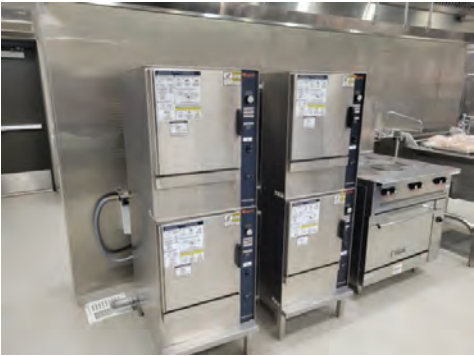
The two existing steamers are not being used. The staff recommends that these units be removed and a conveyor pizza oven be installed at this location.
