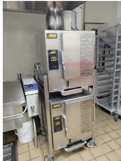
The existing steamers are not being used. The staff recommended removing and replacing these units with a two or four burner range.
