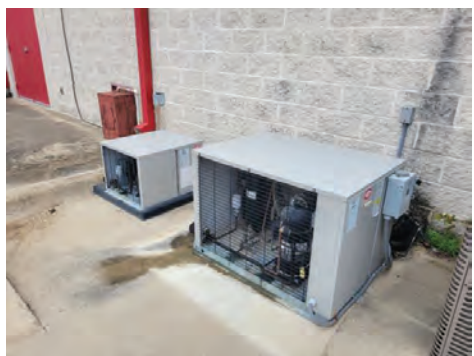
The existing condensing units for the cooler and freezer appear to be in good condition.
