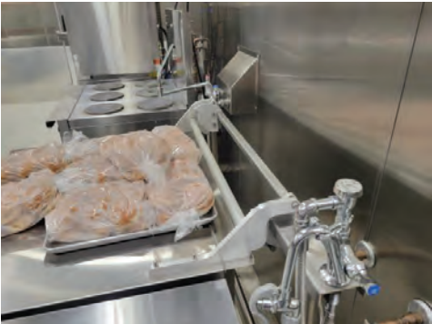
The staff requested that a pot filler with a spray head assembly be installed at the braising pan to assist with the daily cleaning of this unit.
