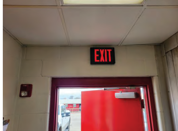
Recommend installing an air curtain above the receiving door to prevent insect infiltration.
