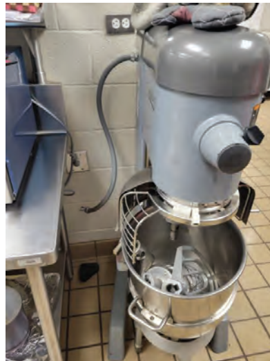
A 208V receptacle and circuit is needed for the 30-quart mixer.
