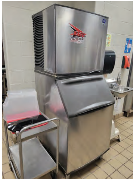
The ice machine was not working and service is needed. Unit appears to be in good condition otherwise.
