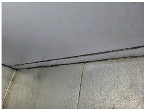
The panel seams in the interior of the cooler and freezer are leaking causing an accumulation of condensation where issue is occurring.
