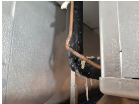
The ceiling penetration around the refrigeration lines in the freezer are not properly sealed.
