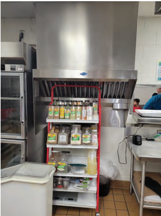
Recommend removing the small existing exhaust hood and providing additional prep table or storage in this area.
