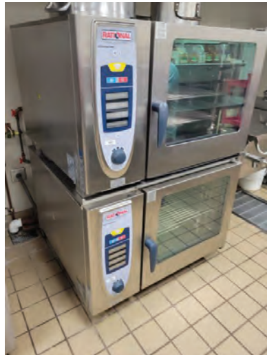
The existing combi oven is having continuous service issues and may be in need of replacement.
